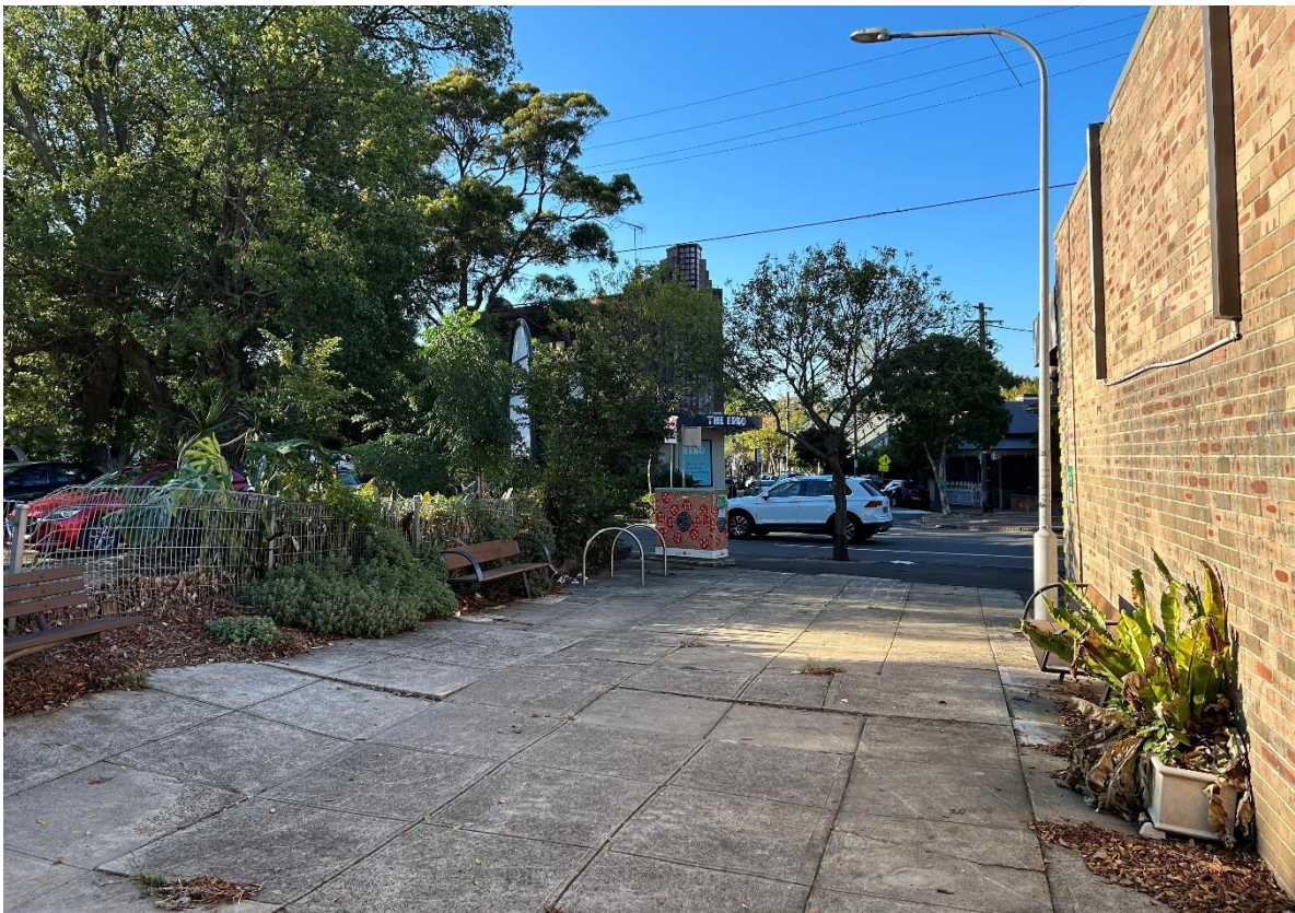
Looking south towards Erskineville Road. Uneven paving and fencing cause by the trees from the neighbouring property which are now removed.
